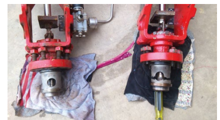
Wear and cavitation of incumbent valves
