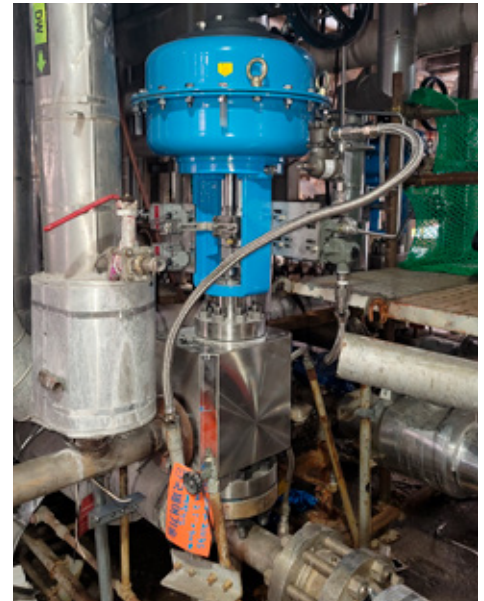
Figure 2: EroSolve MMT valve in service in the petrochemical plant
