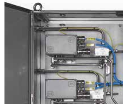
Detailed view of FT Positioners inside control panel
