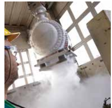
66" cl. 150 actuated after cryo test
